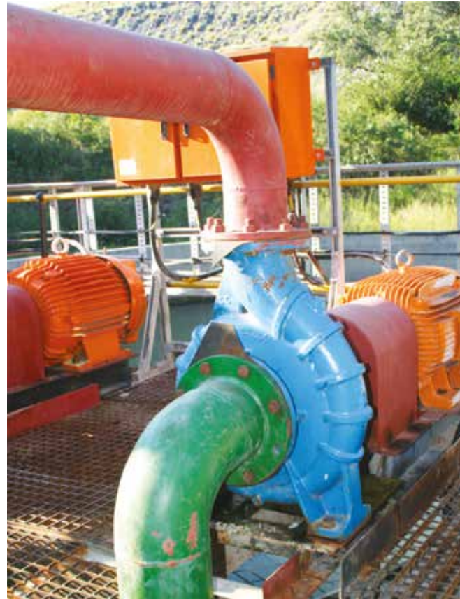
NT Pump Station
