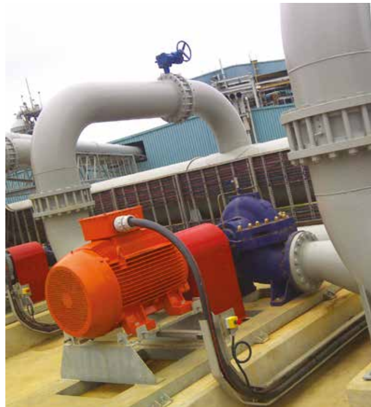
Kwa-Zulu Natal - Evaporative Cooling Plant
